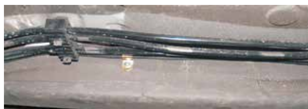
Fig. 8 Autogas line installed with special plates
